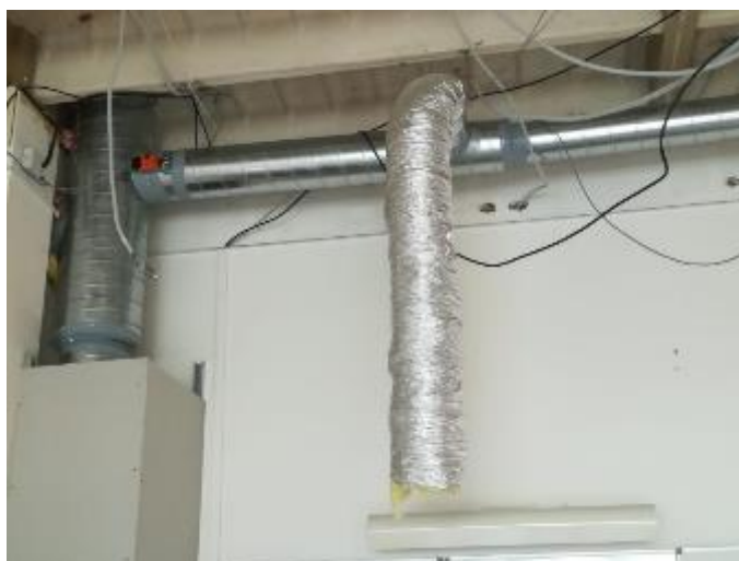
Figure 70 – Installation of a mechanical ventilation system in building N of high school Dautet
