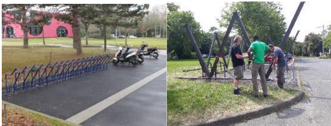
Figure 34 – left: new spaces for bikes and motorbikes, right: construction of a wooden bike shed
