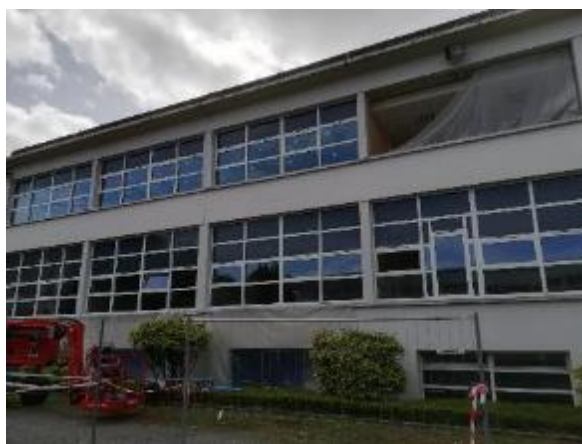
Figure 74 – Replacement of single glazing windows by double glazing windows in building N of high school Dautet
